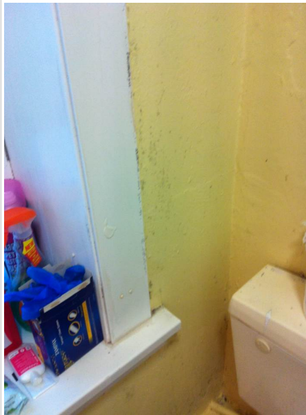
Mould appearing on walls
